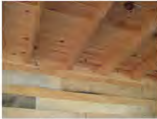
No joist hangers.
