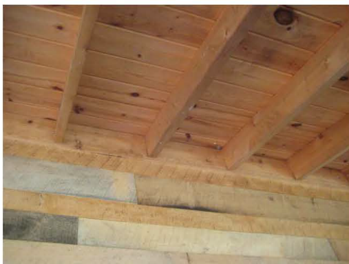
No joist hangers.
