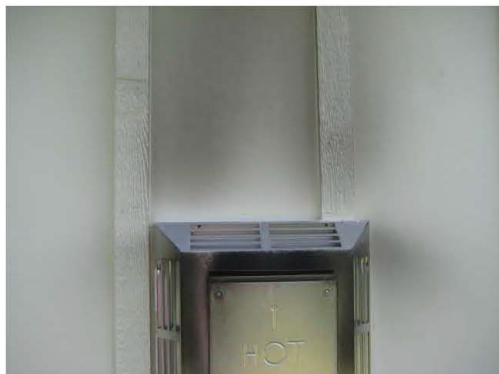
Dark marks on the siding from the fireplace flue.
