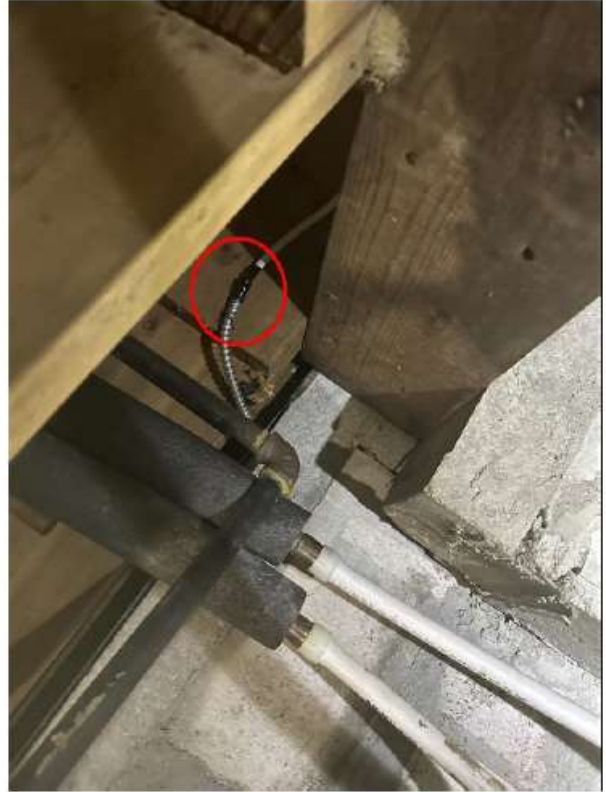
2.3 Item 6 (Picture) open wire splice
