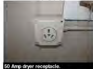
50 Amp dryer receptacle.
