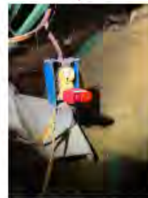
Multiple outlets had no power in attic
