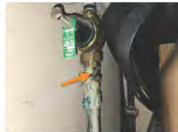
Closer Near Main Valve
