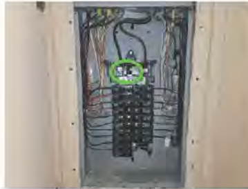
Main Power Shut Off
