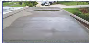
Rolled roofing, standing water main
