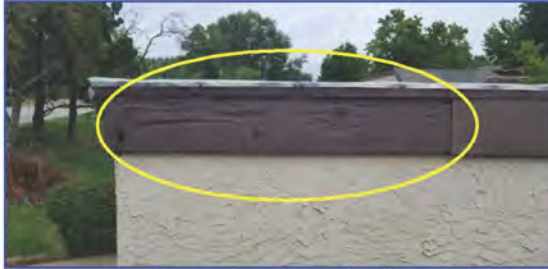
Water damage, rear north facing
