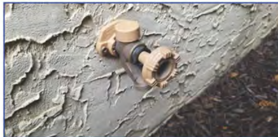
Found in on position, no water
