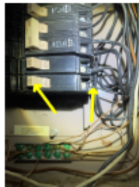
20 amp breaker feeding 14 gauge wire
