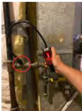
Furnace shut off valve
