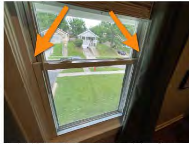
Unit(s)2. won't stay open. Living Room window near Laundry Room
