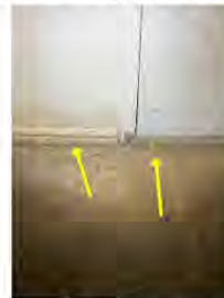
Evidence of moisture intrusion at front wall of basement.
