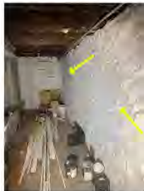
Evidence of movement at left wall of foundation.
