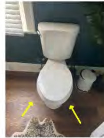
Loose toilet at hall bathroom.
