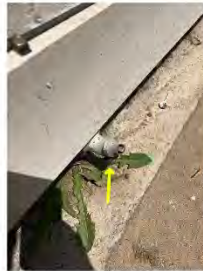
Exterior faucet missing handle at right side of home.
