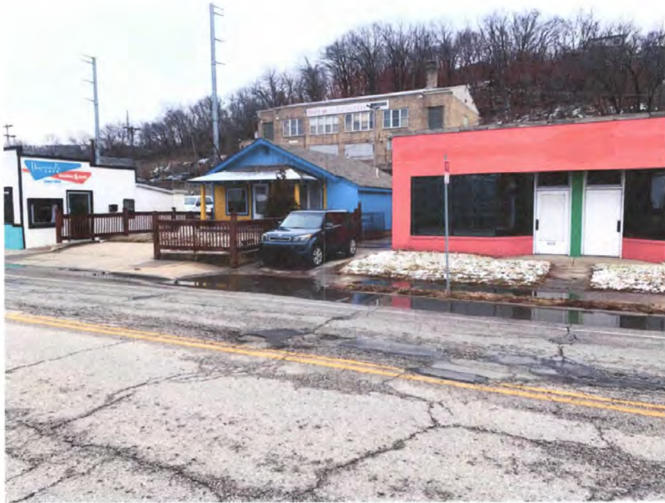
Extent of stormwater curb side puddle resulting from 1 inch of snow January 26, 2023. Two inches of rain has puddled as far left as mid Dagwood's.
