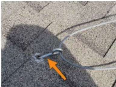
Anchor detached from roof
