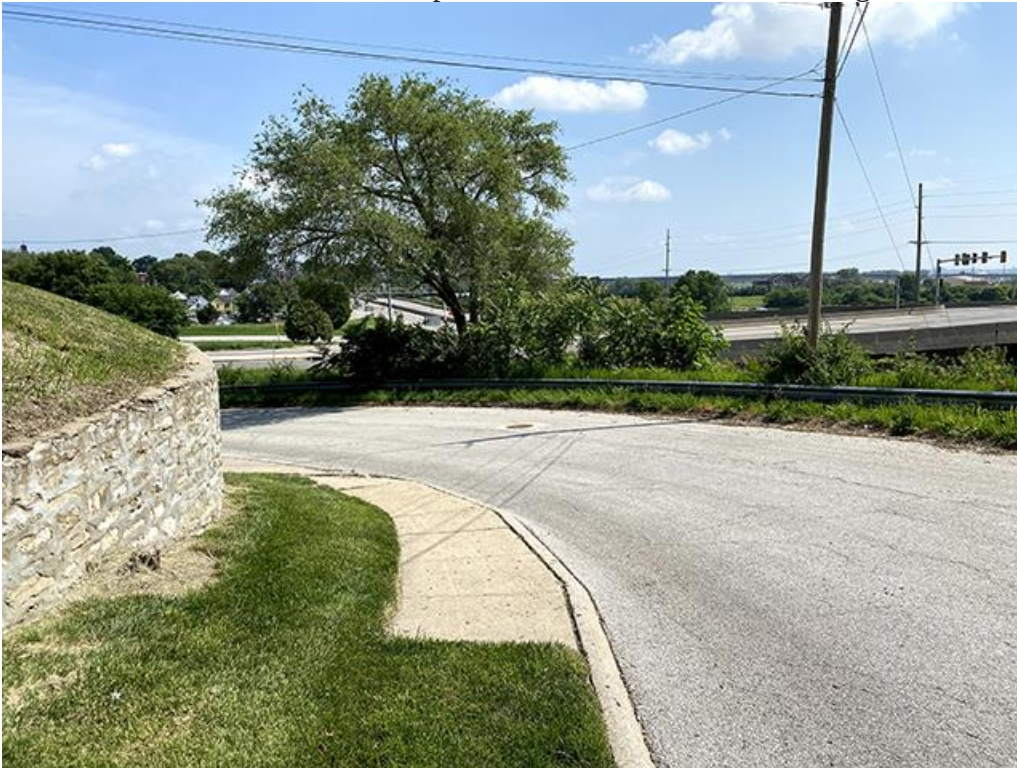
Photo 04: Deterioration of site improvements – Sidewalk ends, overgrown weeds
