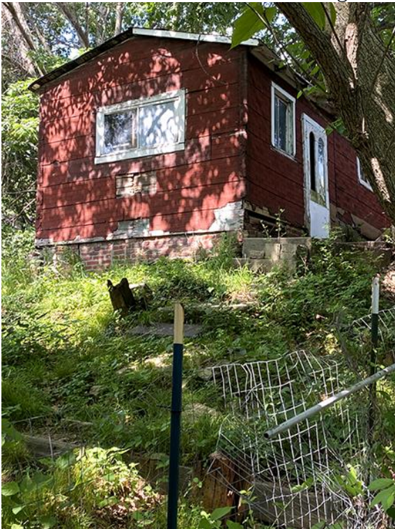
Photo 08: Deteriorated or deteriorating structures, unsanitary or unsafe conditions
