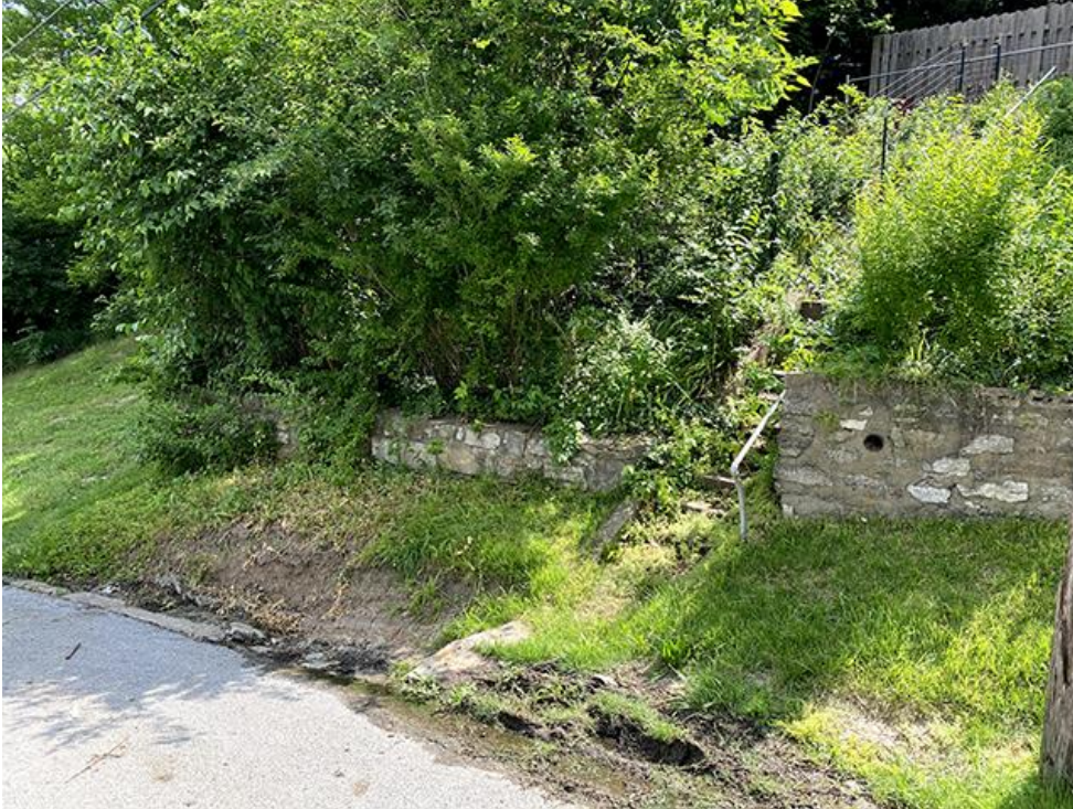
Photo 11: Deterioration of site improvements - No sidewalks, overgrown weeds, erosion, abandoned stairway, deteriorating retaining wall
