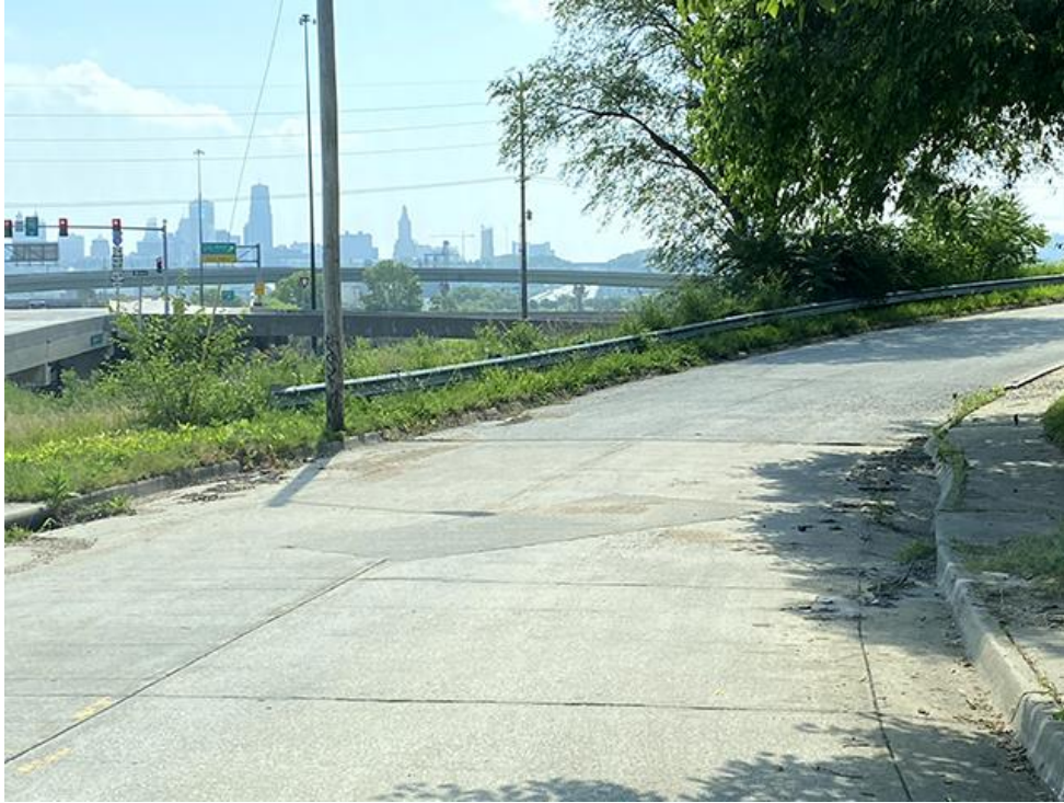
Photo 01: Unsanitary or unsafe conditions – Flooding, debris, overgrown weeds
