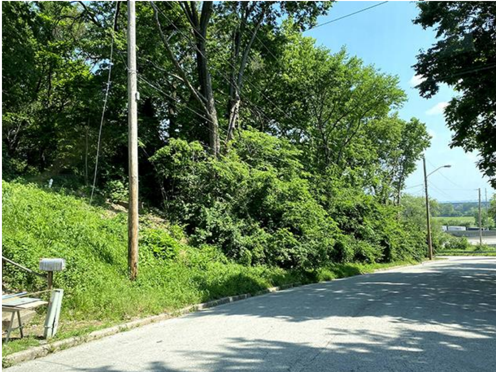
Photo 02: Deterioration of site improvements - No sidewalks, overgrown weeds; deteriorating curbs
