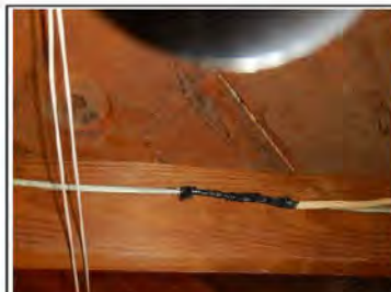
Open wire splice
