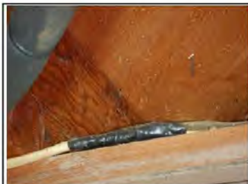
Open wire splice
