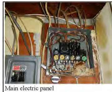
Main electric panel
