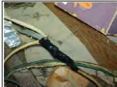
Open wire splice
