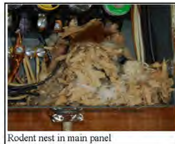
Rodent nest in main panel
