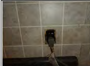
Missing cover plate
