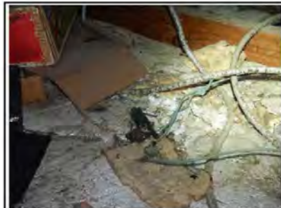
Open wire splice
