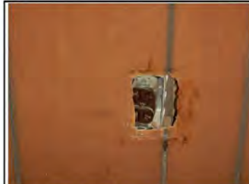
Missing cover plate
