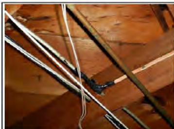
Open wire splice
