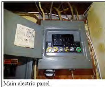
Main electric panel
