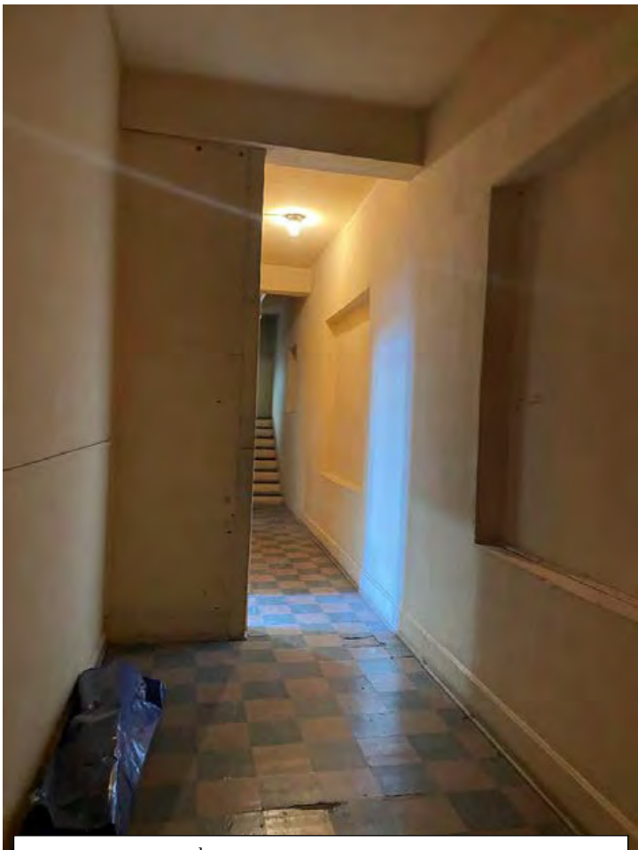
Hallway on 2 nd floor—note the covered windows.
