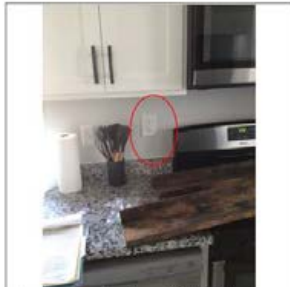
-Proper operational GFCI in kitchen.
