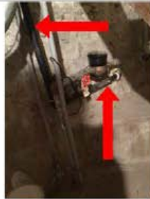
Example of black iron gas line
