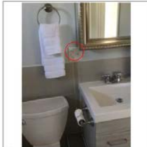
Bathroom GFCI outlets operational
