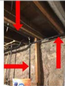
Example of black iron gas line
