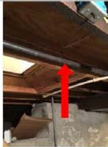
Example of black iron gas line
