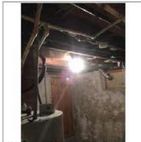
Smoke detector and carbon monoxide detector in basement.
