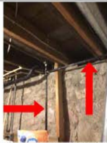
Example of black iron gas line
