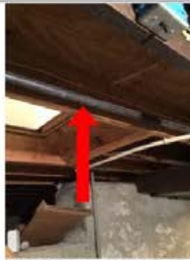
Example of black iron gas line
