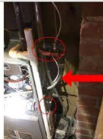
Furnace shut offs
