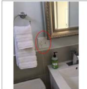
Bathroom GFCI outlets operational
