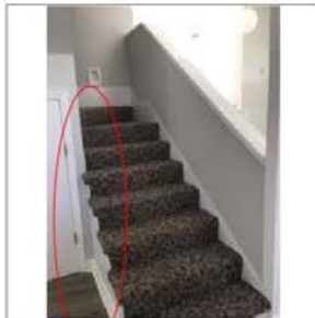
Steps up to 2nd floor Missing railing
