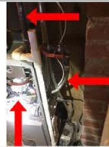
Non bonded CSST gas line , Recommended.
