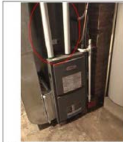
Furnace with proper PVC venting for high efficiency units
