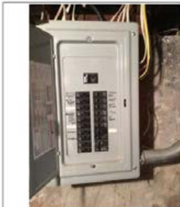
Tape removed from breakers.
