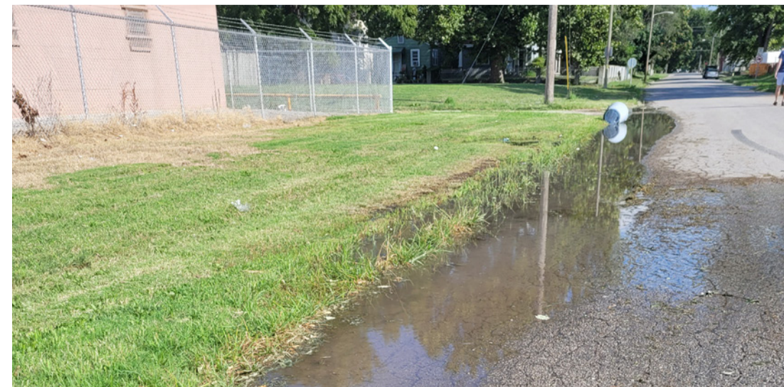
Above: Flooding on Kansas Ave. During Rain Event (YouTube)
