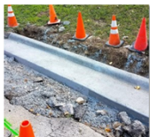
PRE-COVID DEFERRED MAINTENANCE
