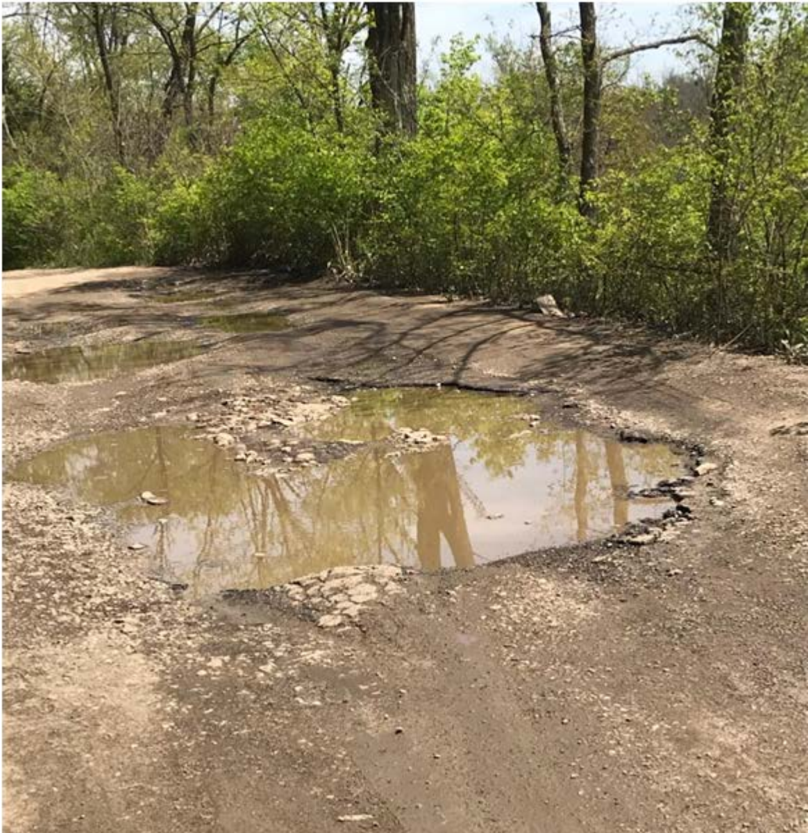
Figure 2: Photograph taken by staff, dated 4/29/2020 showing poor road conditions on Emmons Drive.
