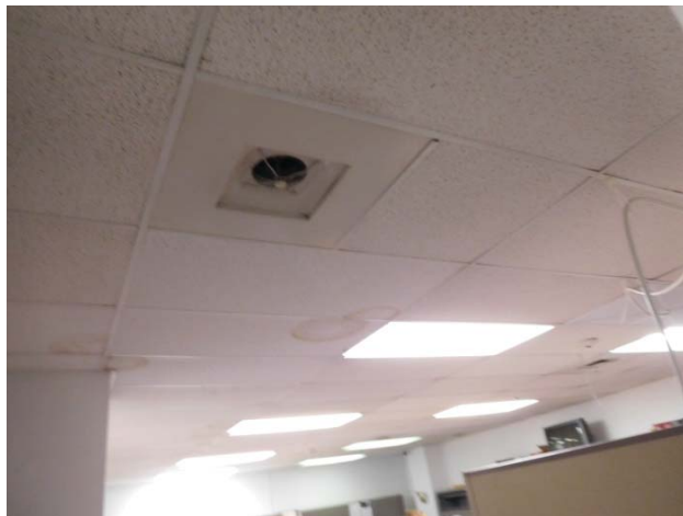
Water damage to ceiling tiles
