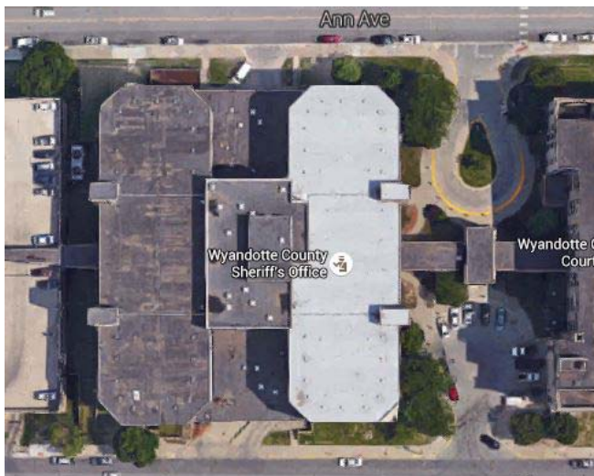
Dark areas of roof in need of replacement
