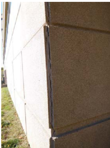
Joint in need of re-caulking
