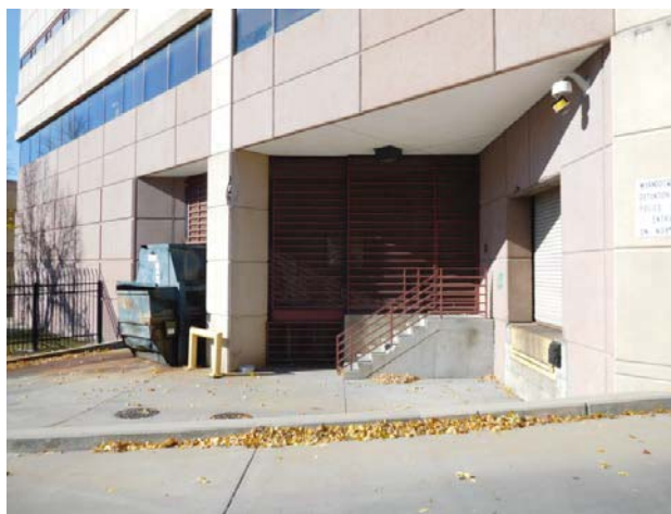
Damage to column near dock
