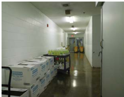
Items stored in corridor
