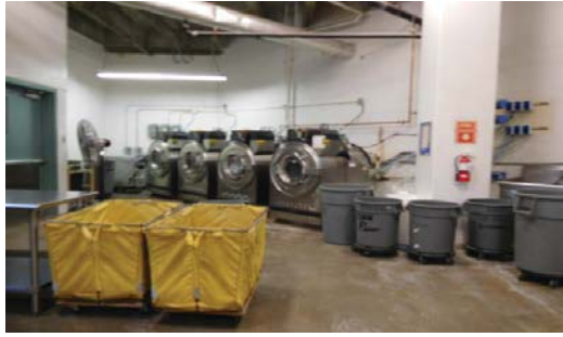
Washers in Laundry Room
