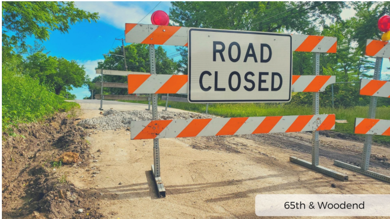
Major road failures due to large rain events washing out the road, making the road collapse.
