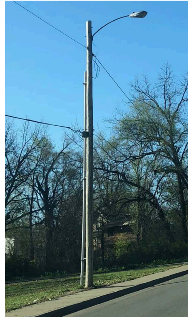
Cobra type lighting fixture typical in the Northeast Area mounted on wooden pole
