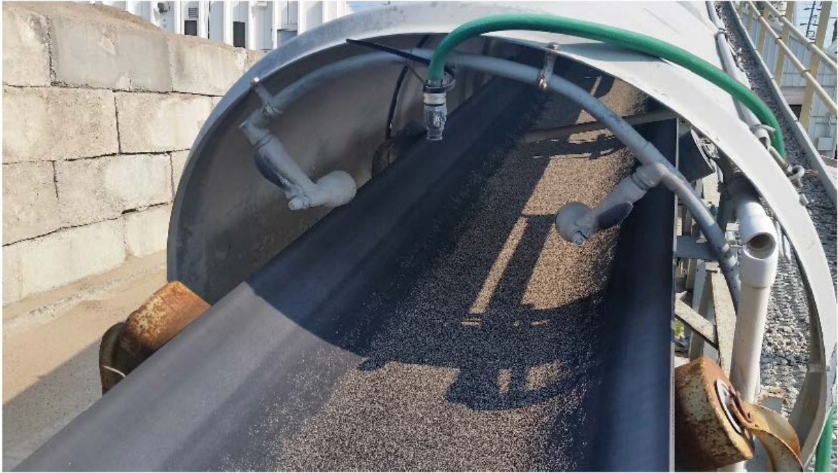
Photo 9-water spray bar to dampen dry rock or sand being conveyed into the plant bins.
