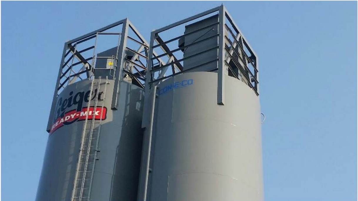
Photo 7-the two large boxes on top of each silo are individual dust collectors.
