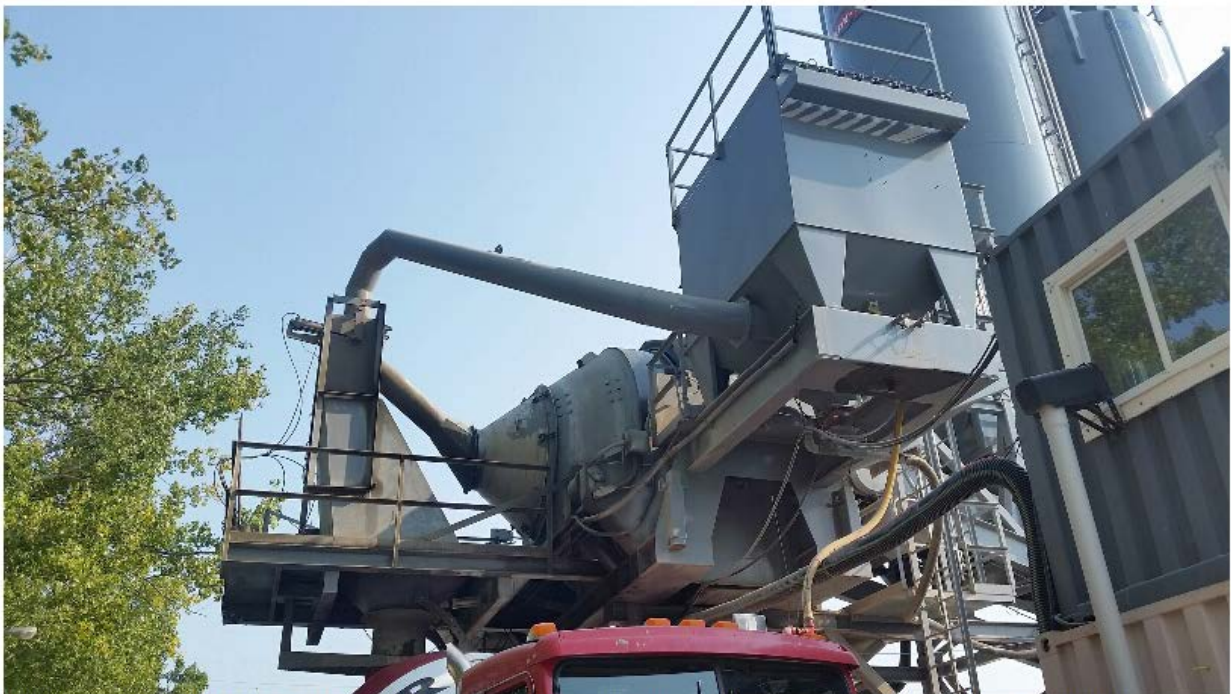
Photo 6-mixer for the wet batch mixing process & shows the central dust collection system and tubing coming off the mixer to the dust collector.
