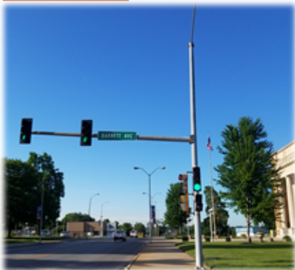
Power coated black poles & LED fixtures
