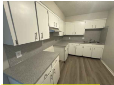
Missing GFCI Throughout Kitchen
