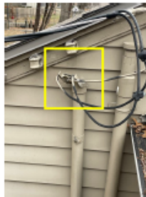
Weatherhead/Mast is damaged
