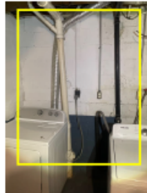
Foundation cracking/movement in basement
