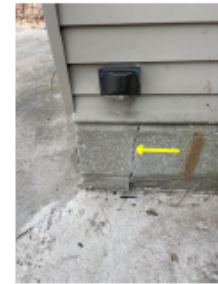
Foundation crack back of house
