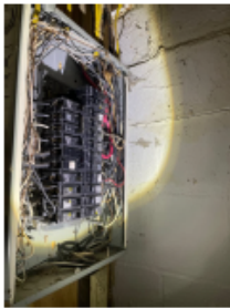
Main panel type = Square D Amperage = 100
