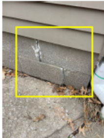
Foundation crack/movement right side of house
