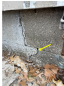
Foundation crack back of house
