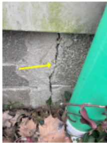
Foundation crack back of house
