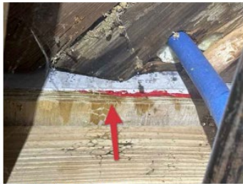
Leaking below shower
