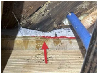
Leaking below shower
