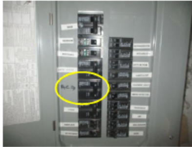
AC unit is on a 30 amp breaker
