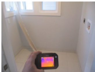
No supply duct in laundry room
