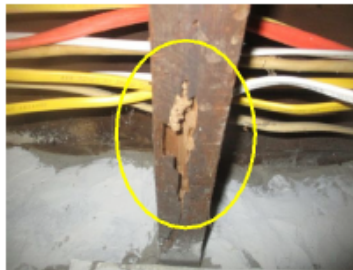
Termite damage on floor joist in basement
