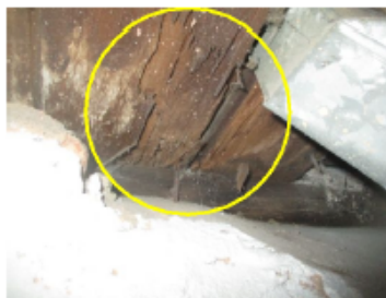
Termite damage on subflooring in basement
