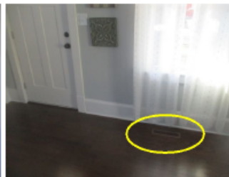
Supply register in living room not connected to duct work
