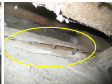
Termite damage on sill plate in basement
