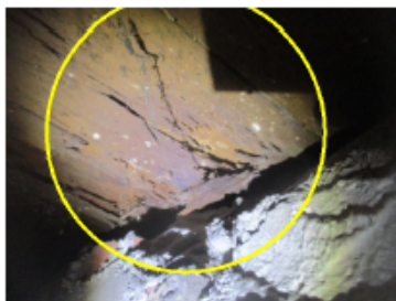
Termite damage on subflooring in basement
