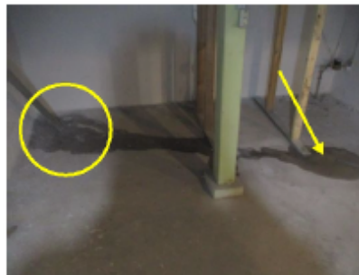
Leaking water from sewer cleanout and floor drain backed up
