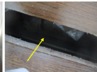
No duct work to supply register near front wall of living room
