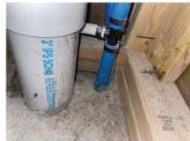
Water coming into house in utility closet (no shut off valve)
